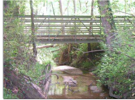
Figure 5. A deeply incised stream crossed by a 26-ft bridge designed by E.T. Techtonics.
