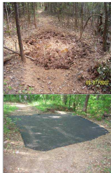
Figure 2. (Top) Boggy spot along the trail caused by accumulation of water in a place with inadequate drainage, (Bottom) geotextiles laid over a boggy spot of the same condition after saturated soils have been removed, ready for the application of crush-n-run.
