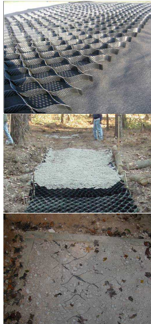
Figure 3. (Top) Geoweb placed on geotextiles, (Middle) Geoweb filled with crush and run, (Bottom) Hardening techniques after completion, with the combination of geoweb, and crush and run.
