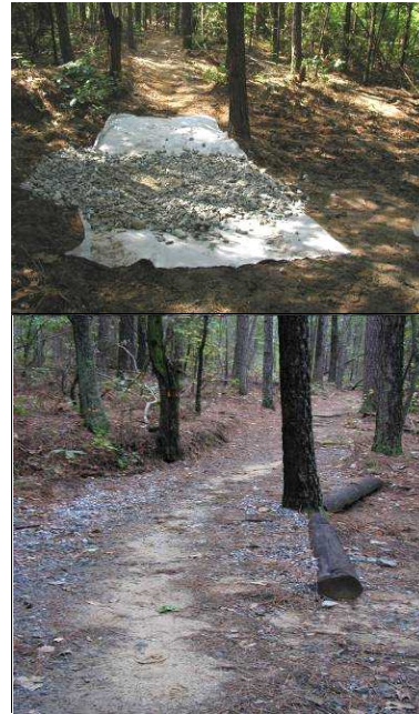
Figure 1. (Top) French drain structure under construction, (Bottom) structure complete, and under use for several
