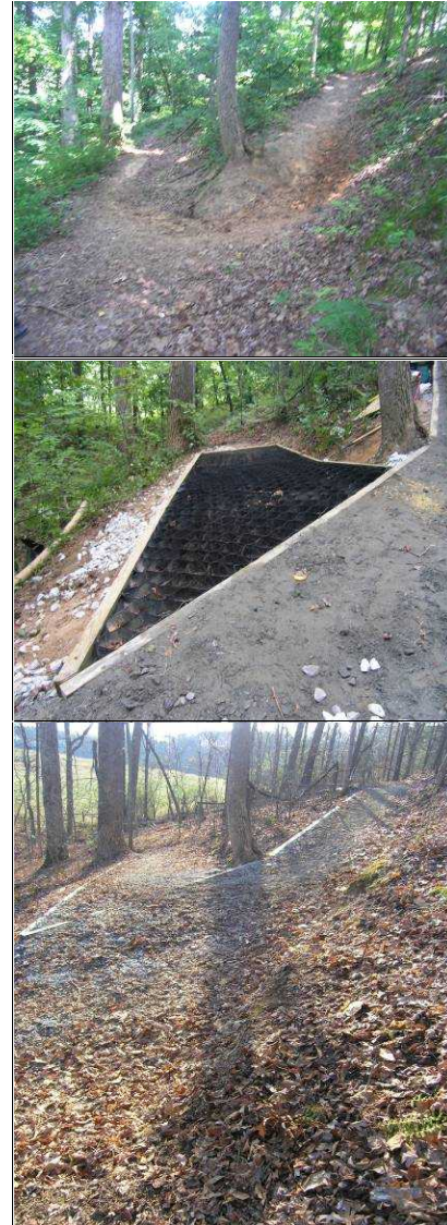
Figure 6. (Top) Erosion in the apex of the turn, caused by users preferring inside of switchback, (Middle) The use of geosynthetics and crush-n-run in the construction of an armored switchback, also shows the out-sloping of the lower leg of the switchback, (Bottom) Several years after construction -- notice an insloping upper leg, and a tree holding the apex of the switchback.
